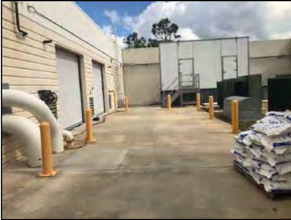
View of South Side of the Building and Generator
