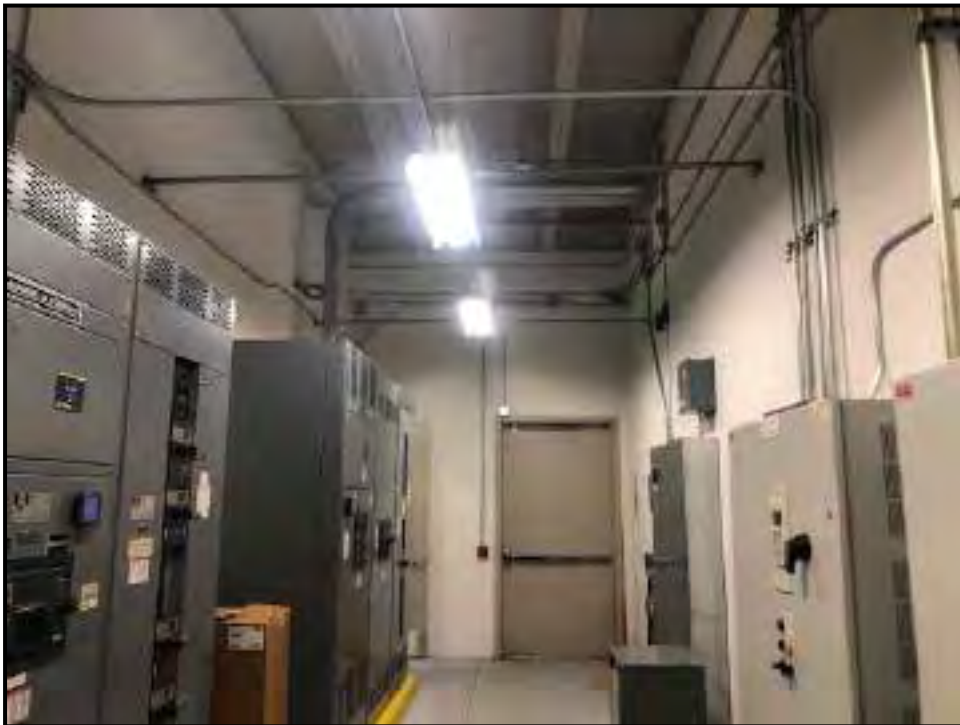
1 st Floor Electrical Room
