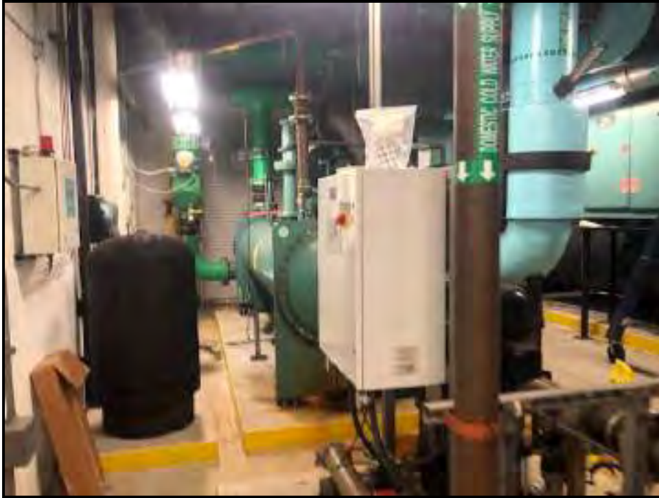
1 st Floor Chiller Room
